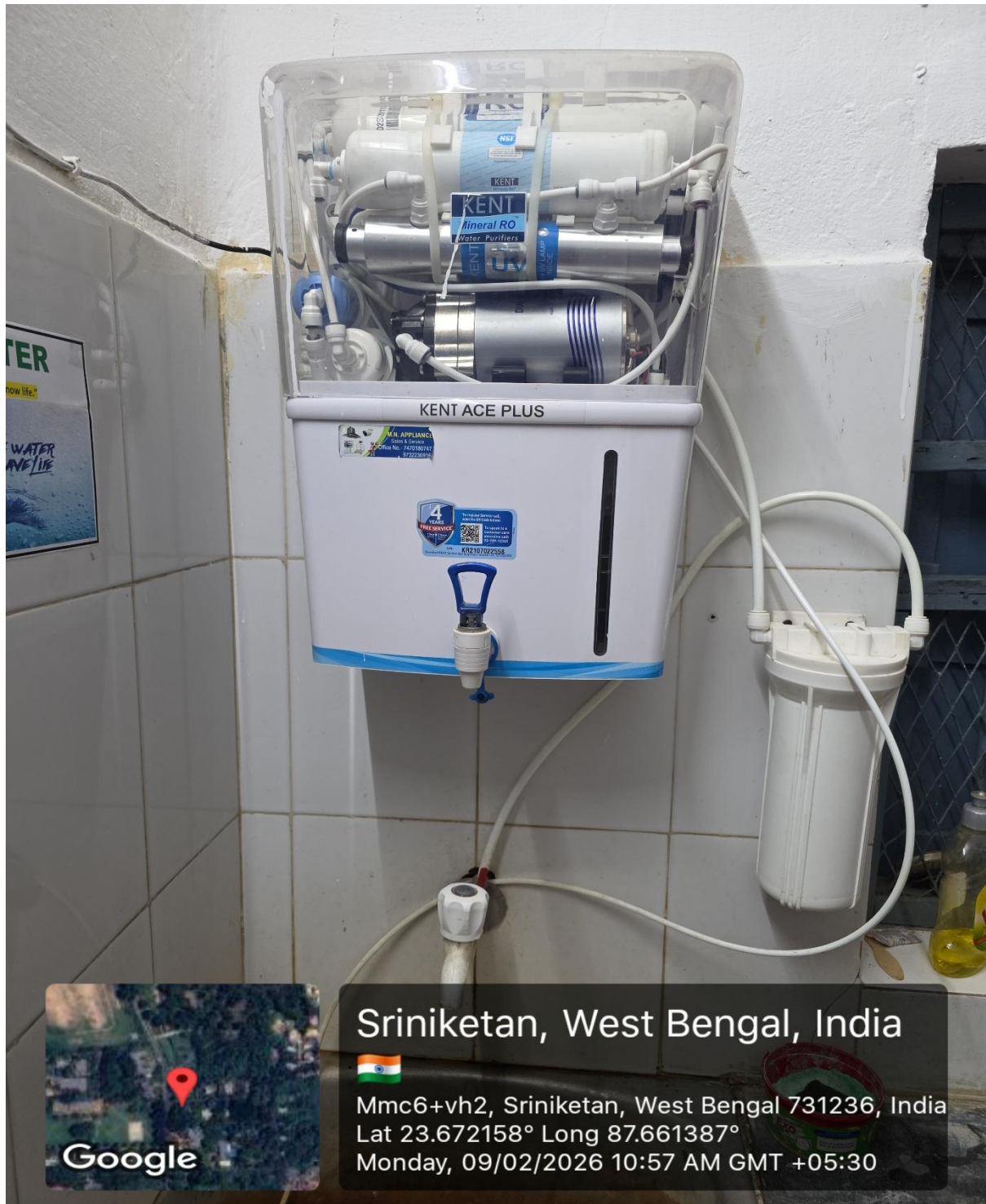
Figure 9: Safe drinking water facility through RO/UV purifier system.
