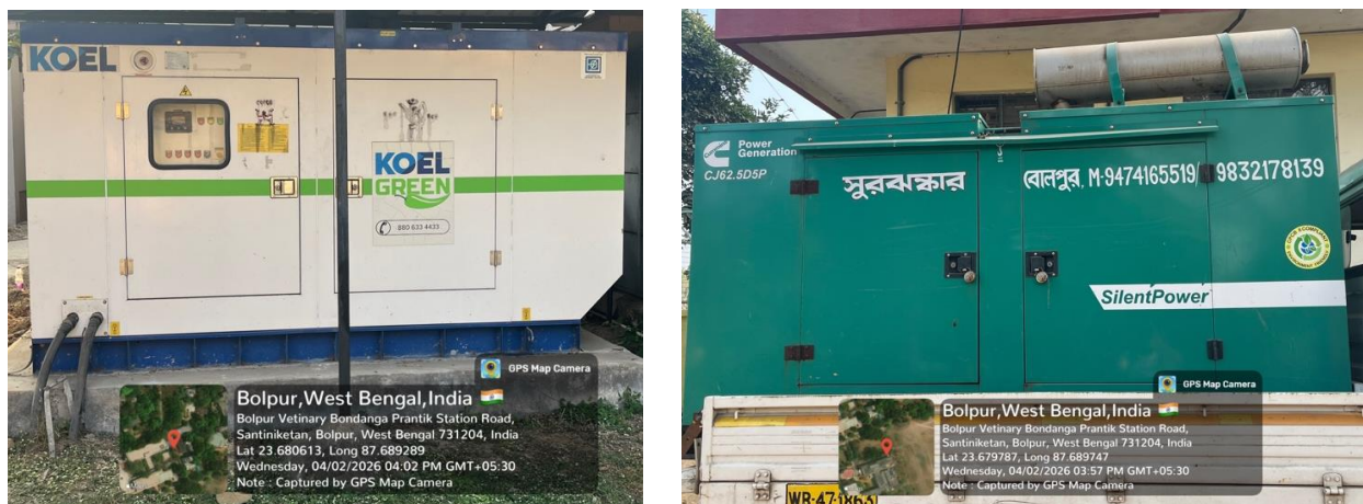
Plate 5: Diesel generators in the campus
